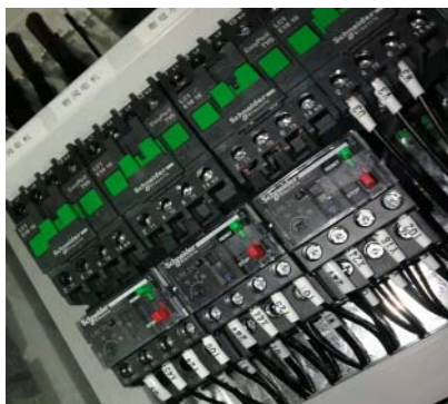
Complete Schneider electric components
